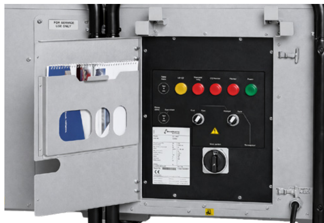
Panel de control
